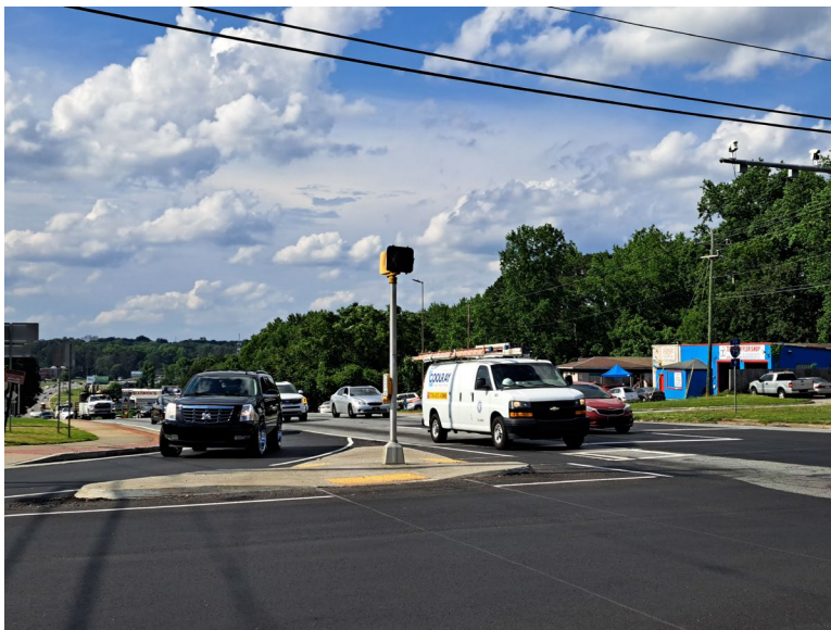
Figure 7-3: View from Austell Road Along South Cobb Drive Show Recent Resurfacing Work
